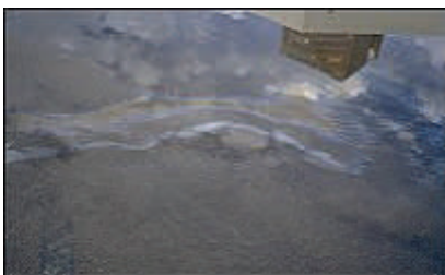
Chemical Contamination and Oil Sheen Indicate a Pollution Pathway
