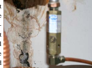
Leaks behind water heaters and plumbing can cause mold growth
