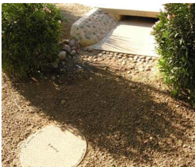
Drywell located in a city designated retention basin
