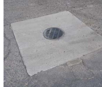
Many drywells are located in vulnerable locations such as recessed loading docks!
