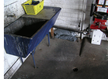
Hazardous/Regulated Materials Improperly Stored Can Contaminate Sub-Surface Soils
