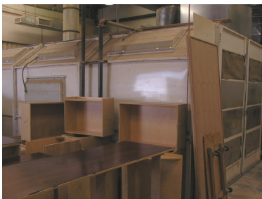
Paint Spray Booths are a Source of Air Emissions
